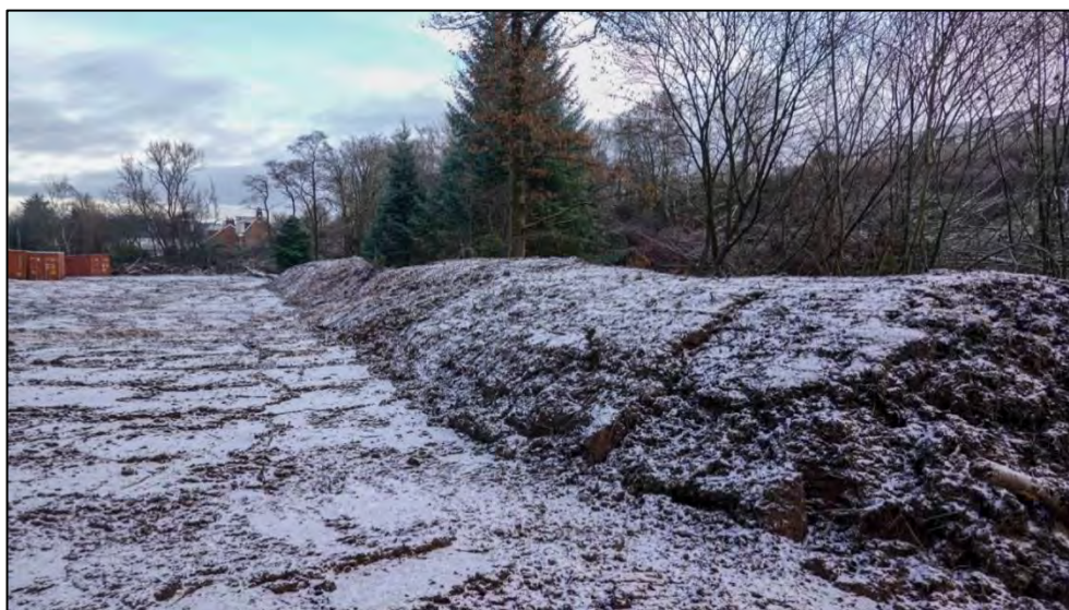
Figure 6: These large soil bunds are just meters from the Bogend Burn and threaten to slump and pollute the watercourse and the entire river Ayr
